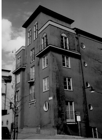
Figure 3 The southeast corner of a 2-year-old building with extensive mould growth of Cladisporium herbarum , a common outdoor mould. The building has exterior insulation with rendering. The growth appears on all 4 sides of the house.
